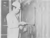
Bollier Inspector R. Amaya visually inspecting welds of wall tubes in No. 7 Tossil boiler.
